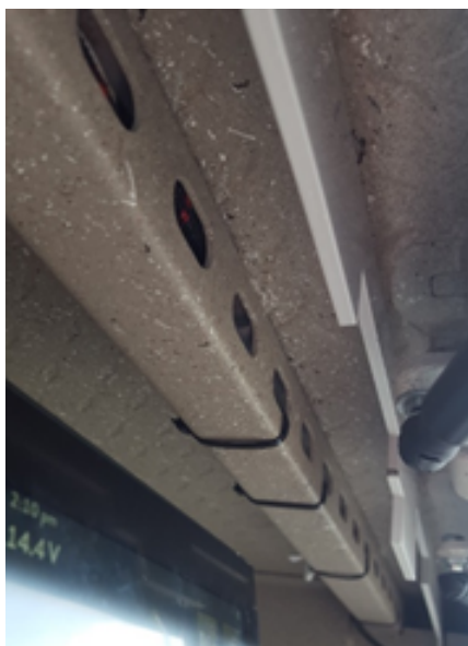
Figure 3 - Secure Channel Wiring
