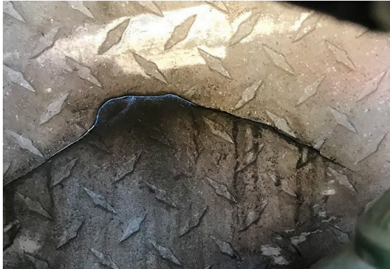
Figure 1 – Sheet Metal Crack
